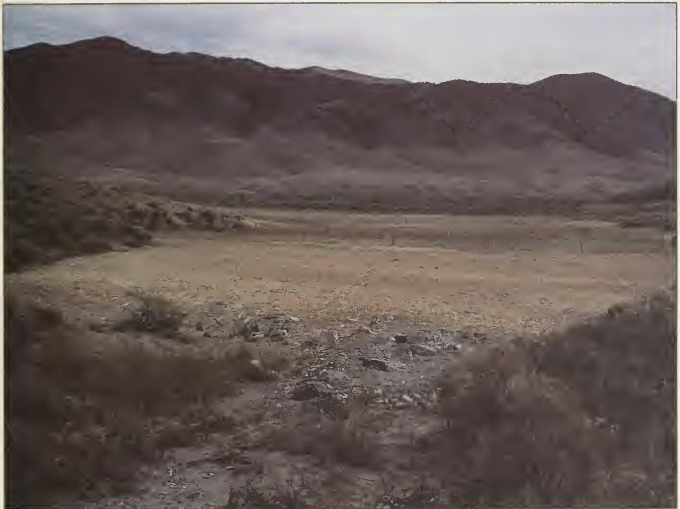
Glen Tungsten Mill site near Dillon, Montana just after reclamation. Straw mulch protects seed which will sprout in the next growing season.
